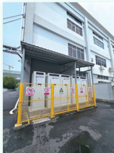
Figure 14. Battery Energy Storage Systems
