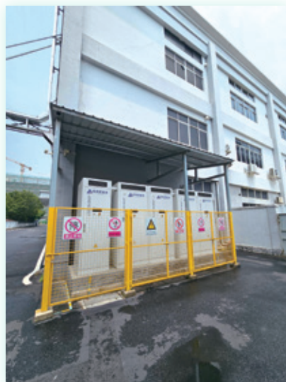
Figure 14. Battery Energy Storage Systems
