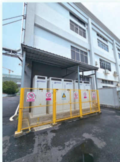
Figure 14. Battery Energy Storage Systems
